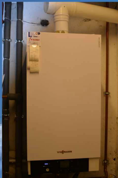
BHKW Vitotwin 300 Fa. Viessmann
